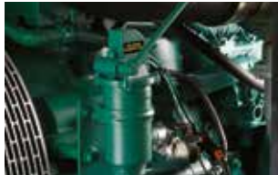
Lube oil drain pump
