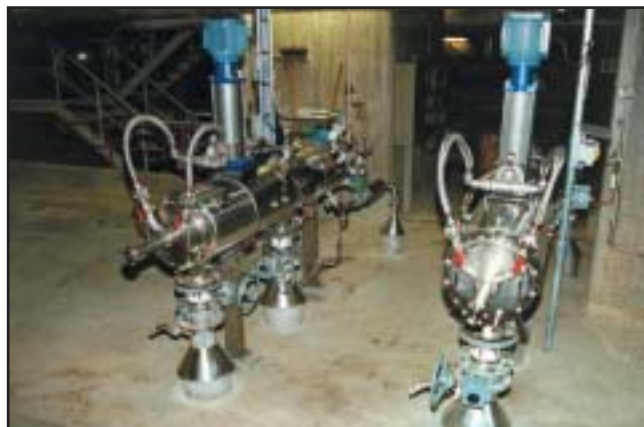
MCFM308XLP paper machine showers - USA
