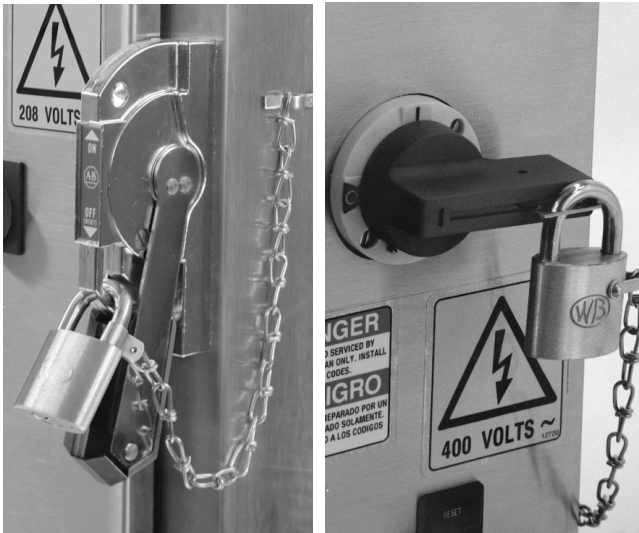
Figure 7 — Power disconnect/lockout switches
