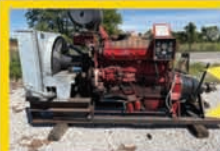
475 HP Cummins Power Unit - Dunnegan, MO
