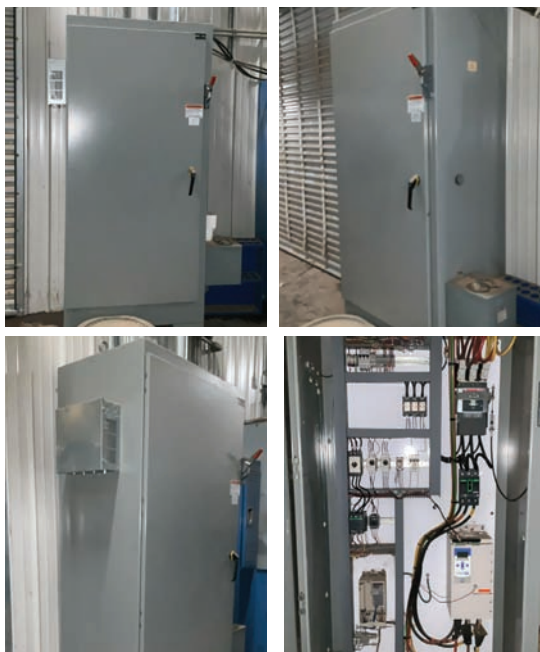
Variable Frequency Drive and Soft Starter for Mill - Dunaway Timber
