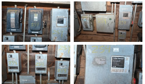
Motor Starters and Disconnects — Description — Includes all starters and disconnects as marked on wall facing Scragg mill, no conduit included
