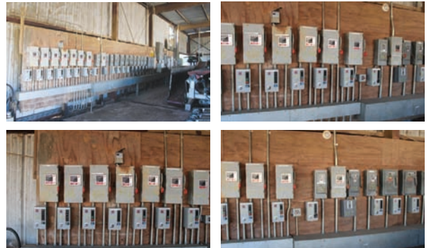
Motor Starters and Disconnects — Description — Includes all starters and disconnects as marked on wall by Jokar Resaw system, no conduit included
