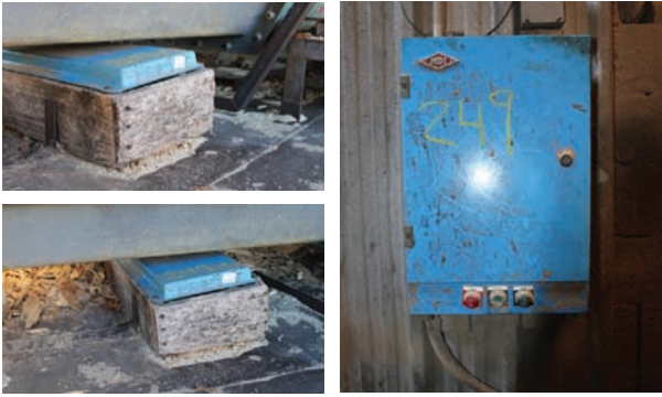
MDI Metal Detector — Description — Includes control panel
