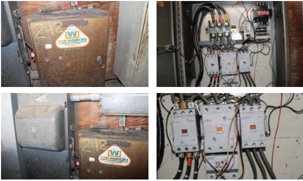
Motor Starter — Description — (Part of an entirety) Metasol motor starter, 400 amp disconnect box
