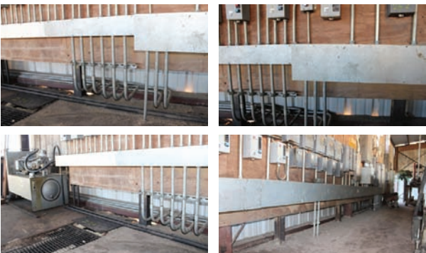
Electrical Wire and Conduit — Description — Includes all conduit and wire from boxes in lot 252, 254 and 256 to equipment, lots marked as 255 and 257 with conduit and wire have been combined with this lot.
