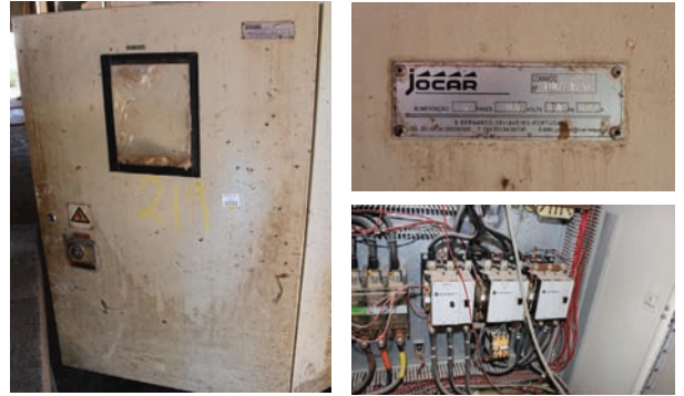
Motor Starters — Description — (Part of an entirety) Jocar 460V motor control panel, includes control panel at end of outfeed rolls
