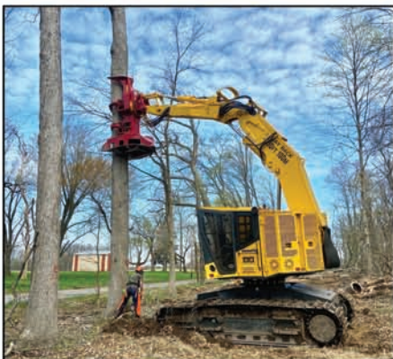
This method of pulling roadside trees is faster, safer, and easier than cabling.
