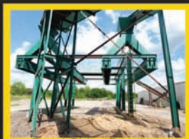
Quad Chip/Sawdust Loading Station
