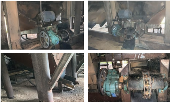
Shop Built Dust Conveyor
