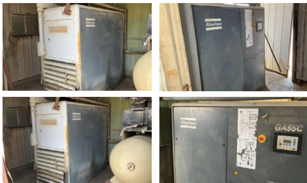
2002 Atlas Copco GA55C Air Compressor
