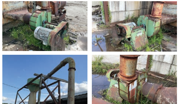
Reckart 22 Dust Blower and Cyclone
