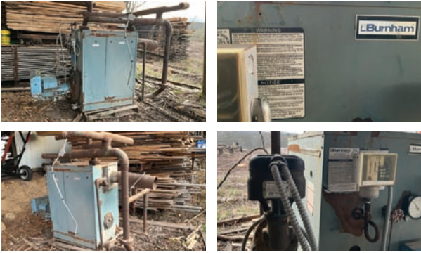
Burnham Water Boiler — Specifications & Features — Year: 1999. Make: Burnham. Model: V-907A. Serial #: 64156650. — Seller Statement — Gas Burner
