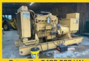
Caterpillar 3406 260 kW Skid-Mounted Diesel Generator Set - Piketon, OH
