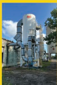
MAC & Dynacom Industrial Dust Collection System
