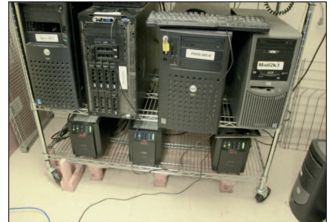
VIEW OF SERVER EQUIPMENT
