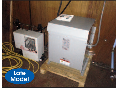
AIR DRYER & TRANSFORMER
