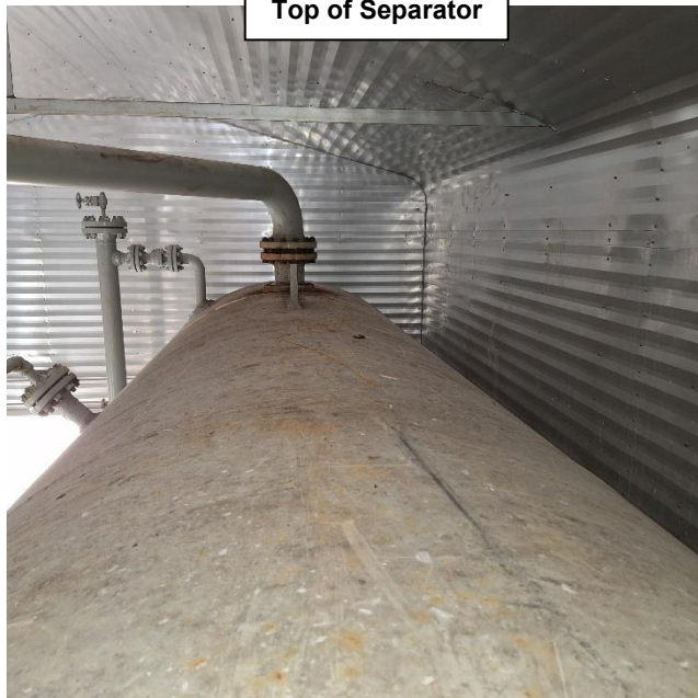
Top of Separator
