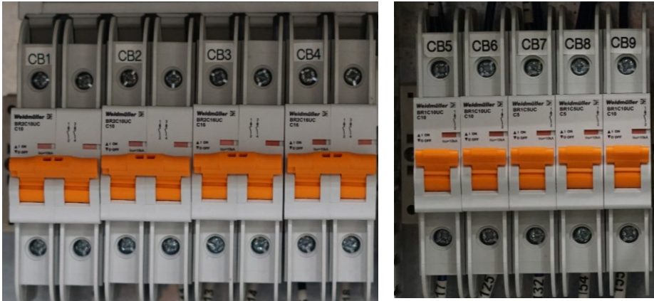
Figure 37 - Circuit Breaker Banks
