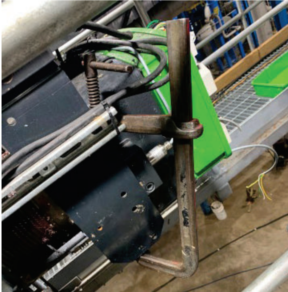
Figure 6-24: Unloading the Load Sensor (Clamp Shown)
