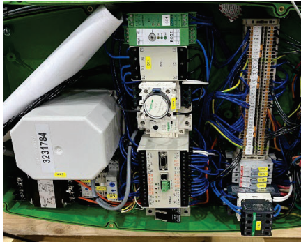
A16 Terminal Box
