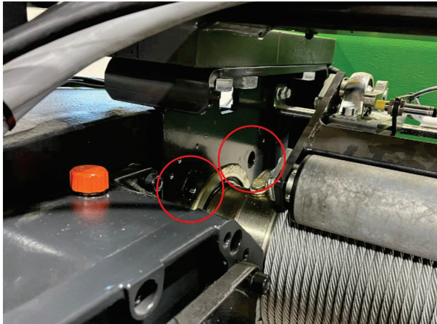
Figure 4-3: Lift Hoist System with Transport Anchor Bolts Removed
