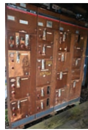
20233 $2,500.00 ELECTRICAL Cutler Hammer 400 amp motor control center, includes various disconnects and starters, good condition 260-633-4047
