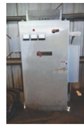
20282 CARRIAGE DRIVE $7,500.00 Jacobson AC/DC, control box w/250A, 600 VAC 460V transformer, 125hp electric motor w/blower motor, includes conduit from boxes to equipment 260-633-4047
