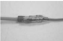
Orange wire connection
