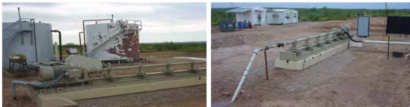
Figure 3: SPS™ Pump Installation
