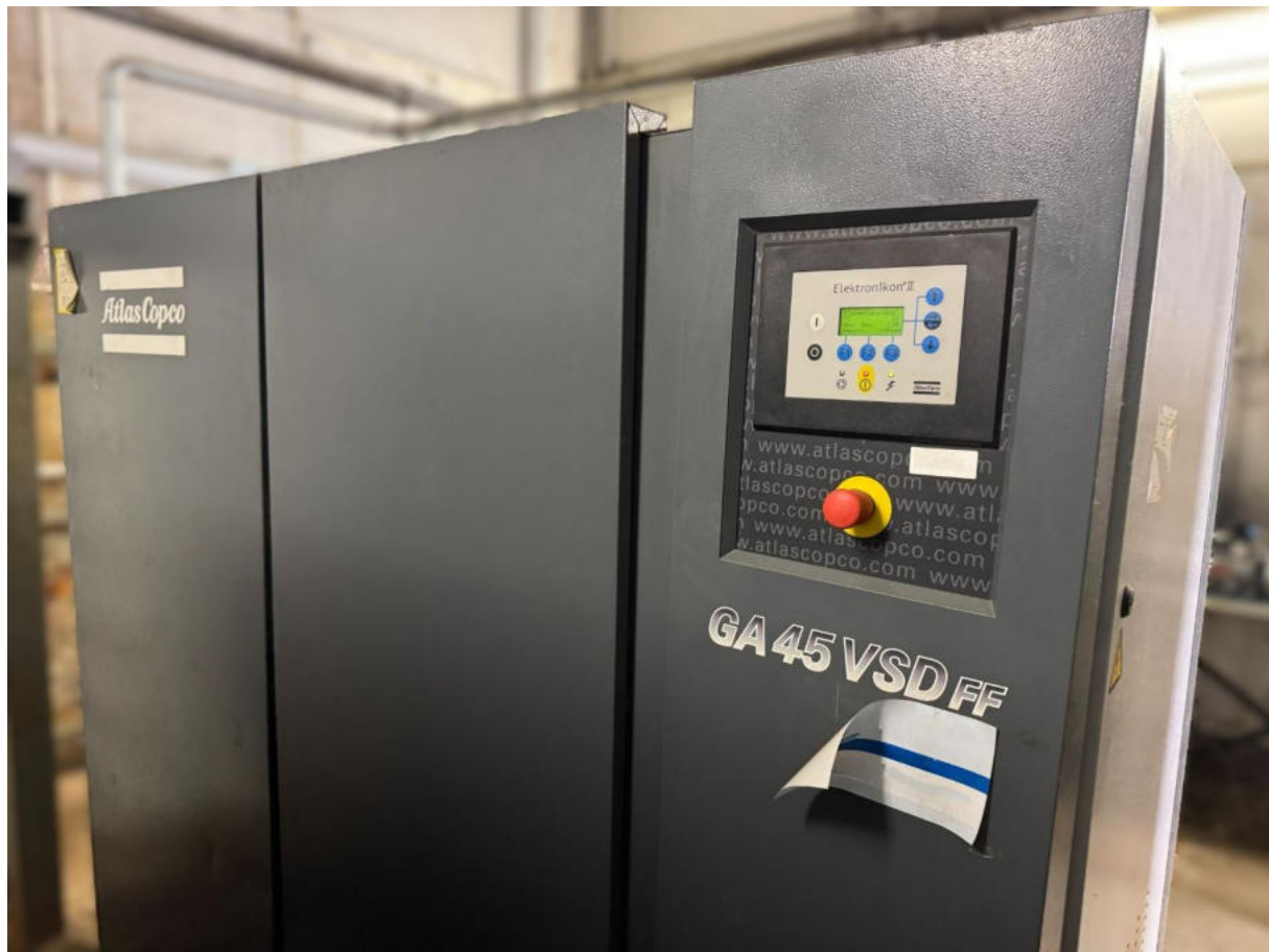
Compressor ATLAS COPCO GA45VSD – 2008
