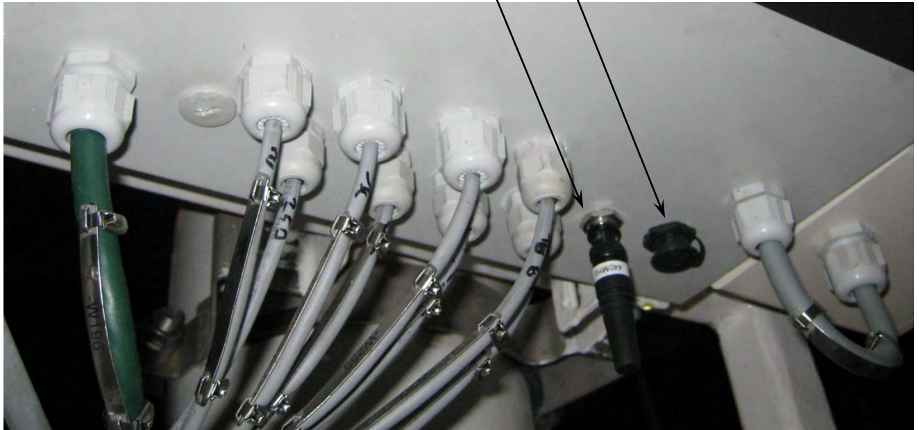
Underside radio remote cabinet –A97 (typical)
