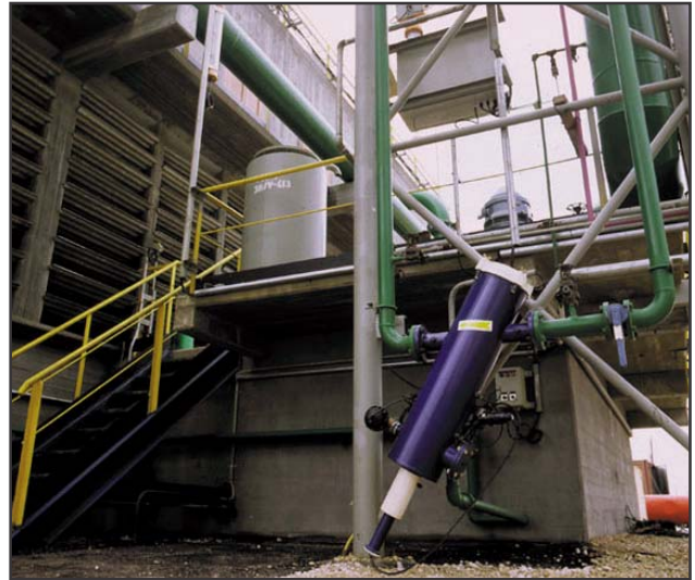
M303L in-line side stream filtration for cooling tower at petro chemical plant - Israel.
