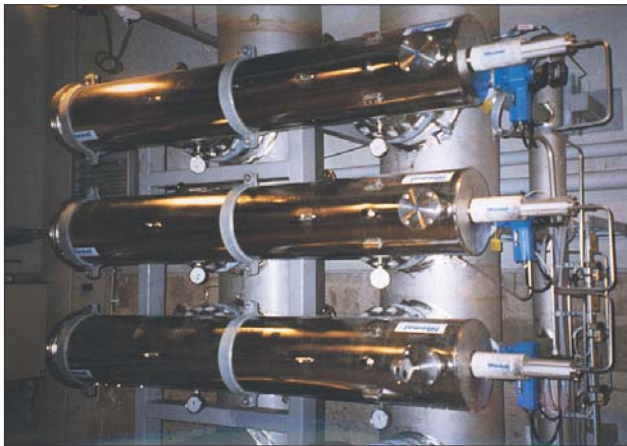
M314P St/St in-take water at paper mill - Finland.
