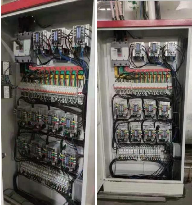
Electric heating control cabinet (not included; to be US-built)
