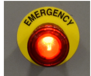
Figure 4-2: Emergency Stop button
