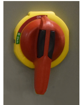
Figure 4-1: Main Power Disconnect Switch
