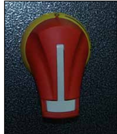
figure 16-1 Main Disconnect Switch
