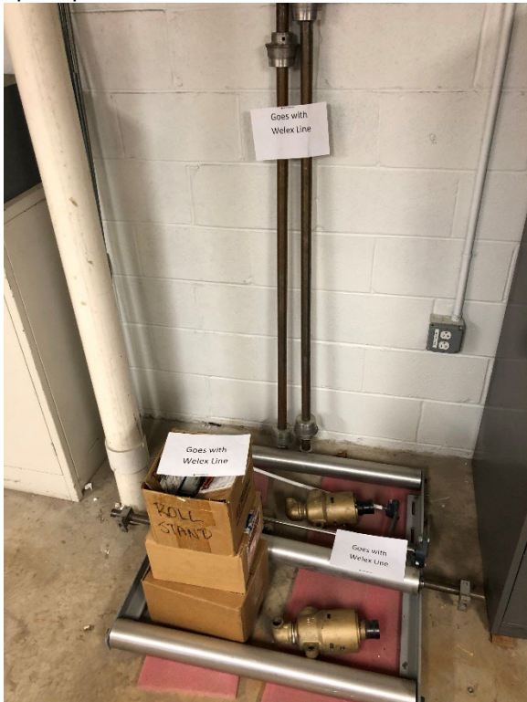
Spare parts and lamination rolls in Mezzanine:
