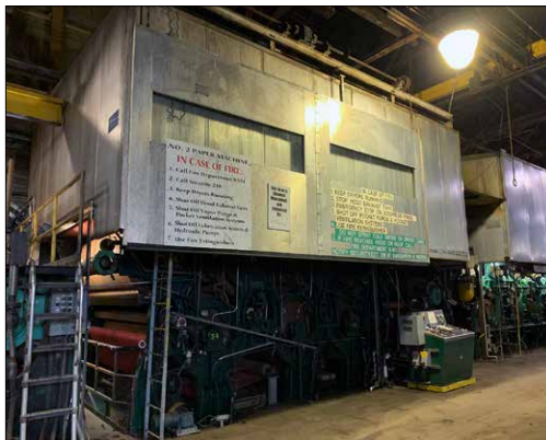
Second Dryer Section
