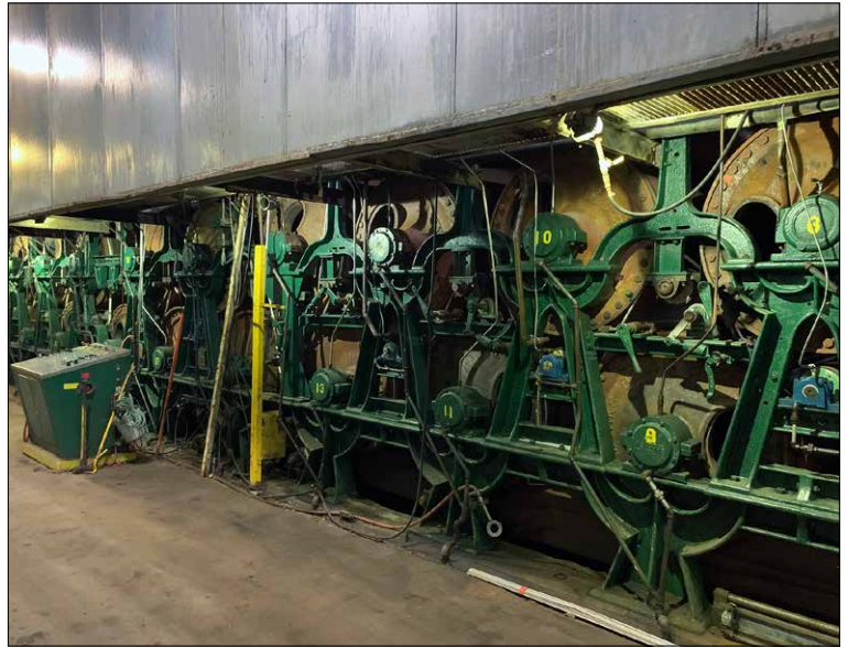
Main Dryer Section
