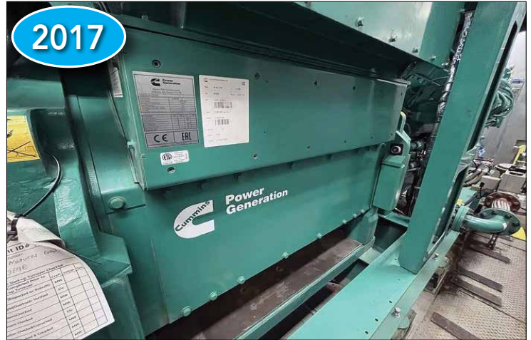
1400 kw Cummins Natural Gas Back Up Generator Set 13,800 Volts
