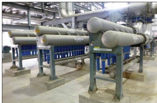
Celleco Cleanpac 350 Cleaning Bank System
