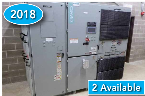
Siemens Perfect Harmony Drive 750 HP
