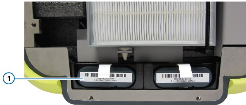
Figure 9-1. Checking the batteries
