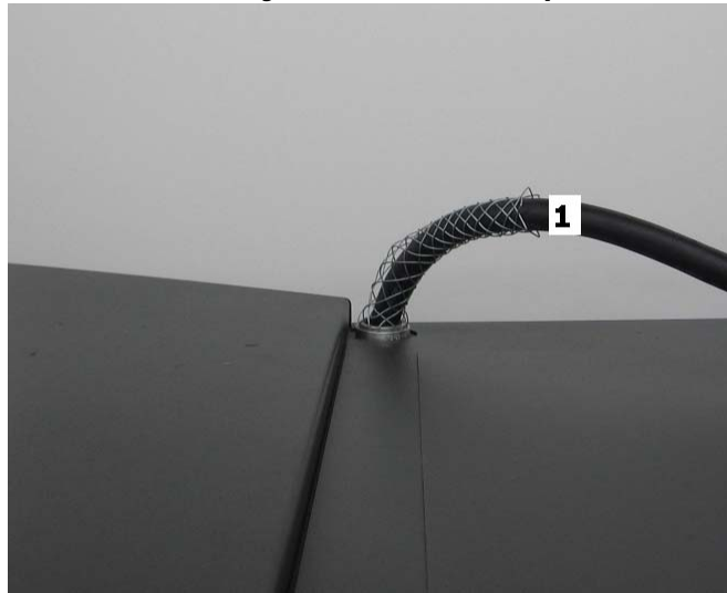
Figure 1-7: AC Power Cord from facility circuit breaker panel, into top right rear of printer
