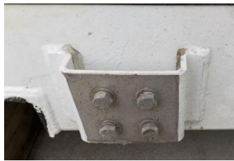
Figure 5-11 Grounding connection point
