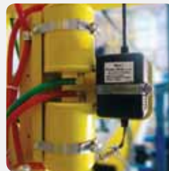
Two vacuum tanks
