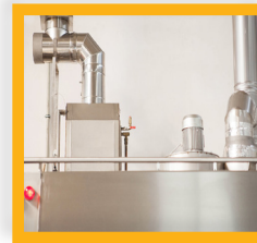
Steam Oven Chimney System
